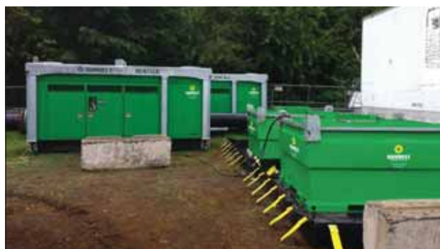
Two containment berms holding auxiliary fuel tanks at a dewatering project in Seattle, WA
