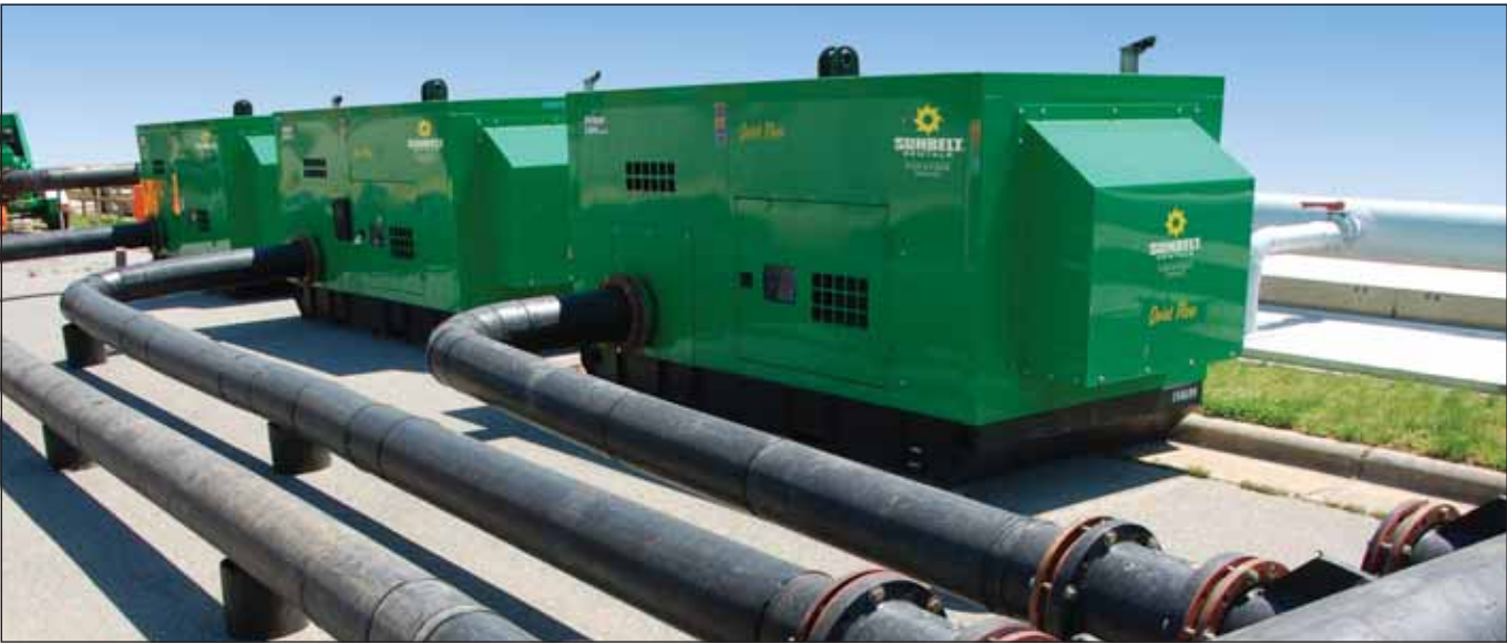
(3) Quiet Flow 12" Silenced Diesel Trash Pumps Working on a sewer bypass project
