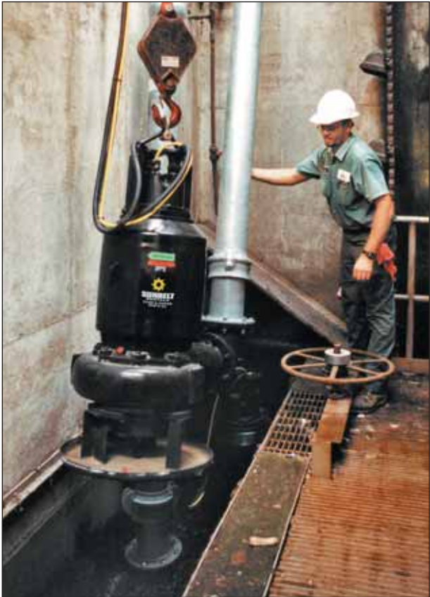
Gorman-Rupp 8" 70 HP Trash Pump One of four 8" trash pumps utilized on a wastewater treatment plant bypass job being lowered into a wet well
