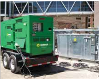
5,000 CFM Electric Desiccant Dehumidifier & 175 kW Generator
