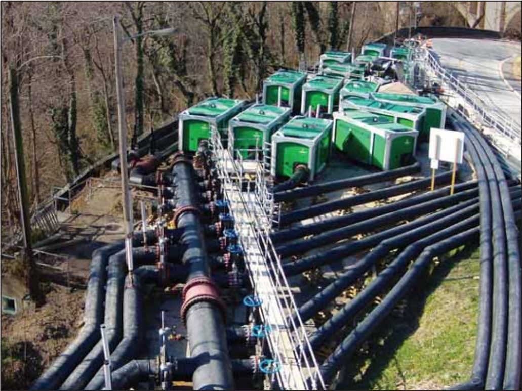
Sewer bypass completed in Baltimore, MD., with 16 18" Quiet Flow™ pumps, all designed and installed by Sunbelt Rentals Pump & Power Services.
