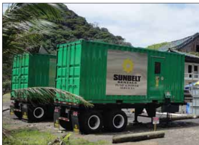
Two paralleled MQ Power 500 kW Generator Emergency power for disaster relief
