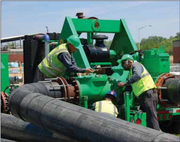
Sunbelt Rentals technicians servicing a 24" diesel trash pump on a multi-pump municipal sewer bypass project
