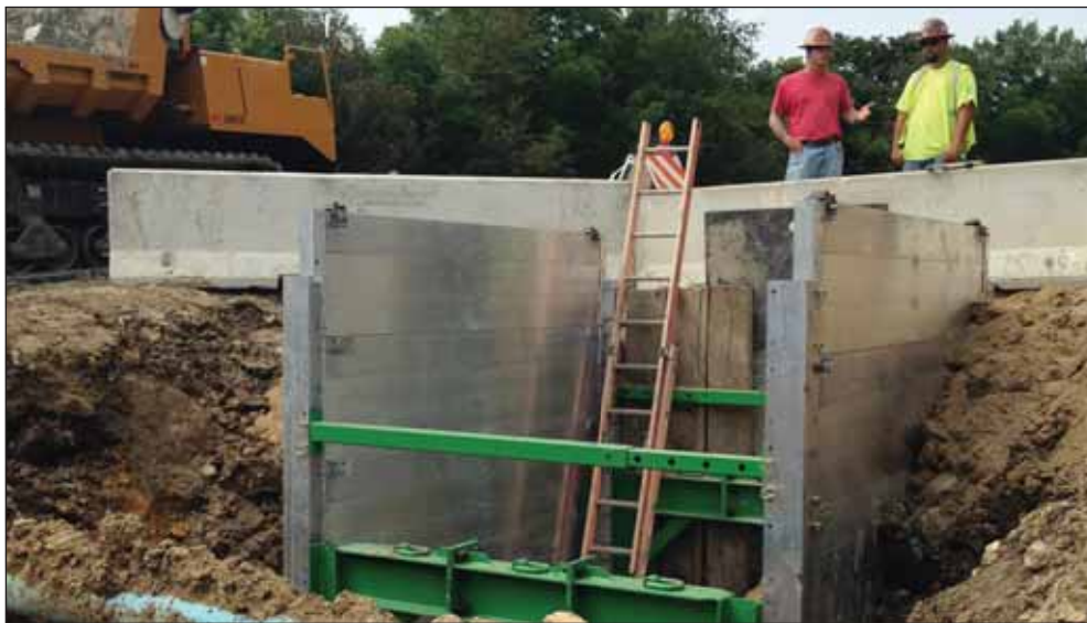
A custom engineered shoring installation on a natural gas transmission line project. Two 8' x 16' 4" wall aluminum trench boxes with 20' steel spreaders were utilized
