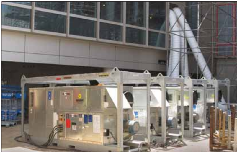
Above: Four 5,000 CFM Electric Desiccant Dehumidifiers in operation at a construction project in CA.
