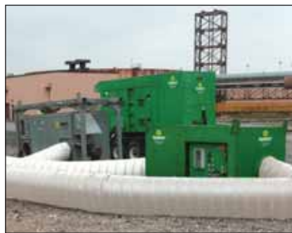
5,000 CFM Desiccant Dehumidifier, 320 kW Generator & 150 kW Heater
