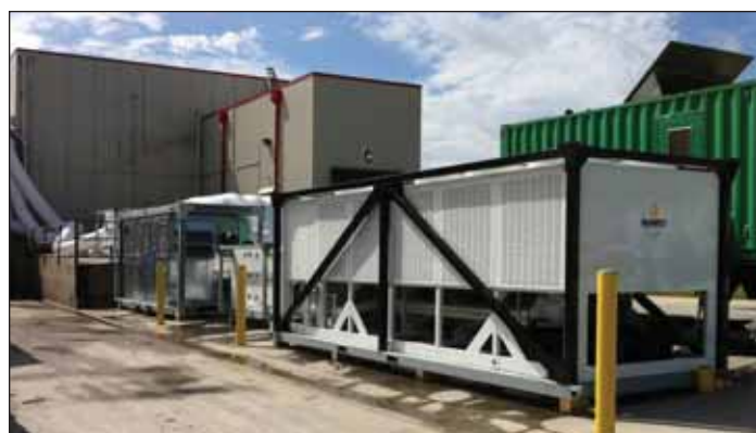
Chiller, air handler and generator at a processing plant
