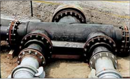
A 24" diameter HDPE manifold combining the flows of (4) 12" discharge lines on a sewer bypass project
