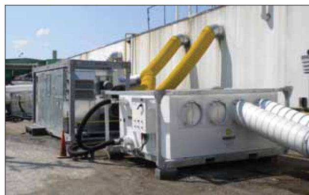
Desiccant dehumidifier and air handler at a processing plant
