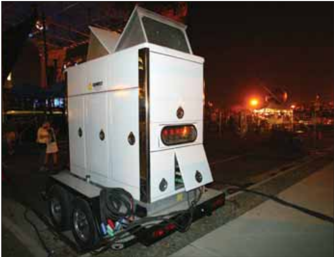
Crawford 1,400 amp Movie Set Generator Powering sound stages at an outdoor concert
