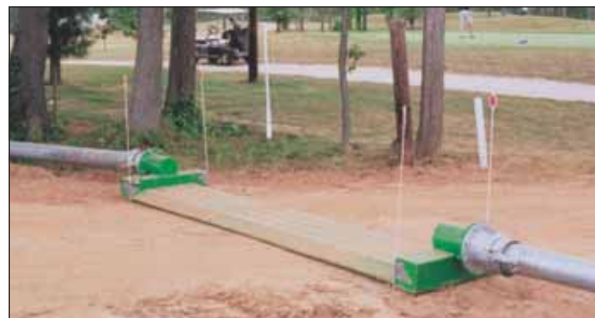
An 8" x 12' road ramp in operation on a golf course drought relief pump project
